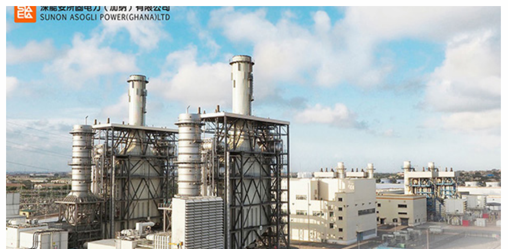
Sunon Asogli Power Plant
