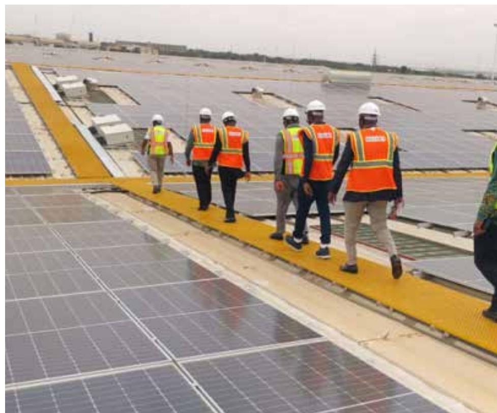
1000 megawatts rooftop solar project
