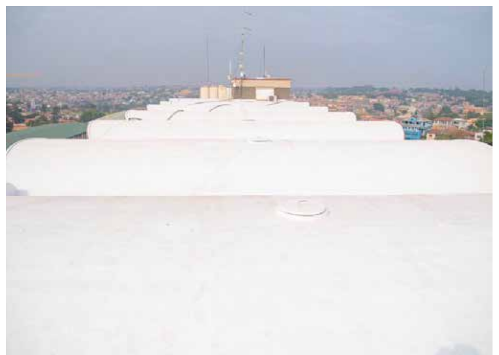
Repaired leaking concrete roofs in the old "Gee" blocks at Komfo Anokye Teaching Hospital (KATH)
